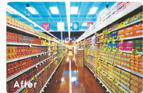
After New T8 LED Retrofit Tube (18W)
